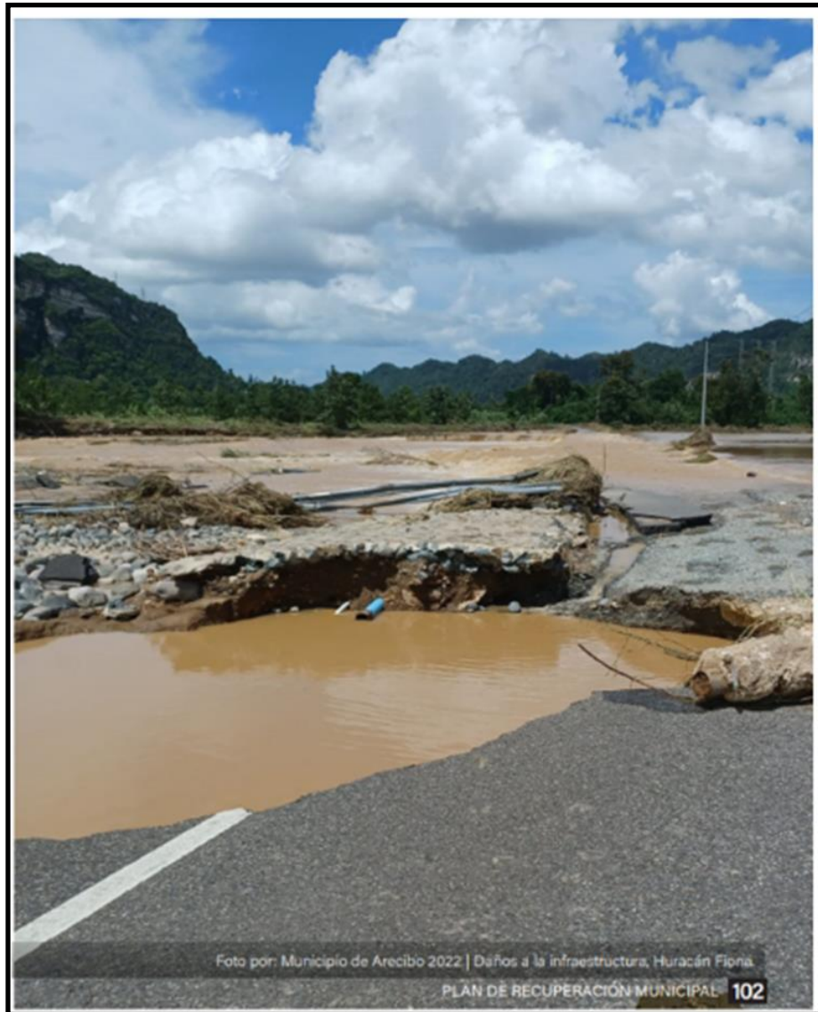
Figure 28: Road Damage near Jurutungo sector and the Río Grande River in the Municipality of Arecibo. MRP Plan Municipality of Arecibo.
