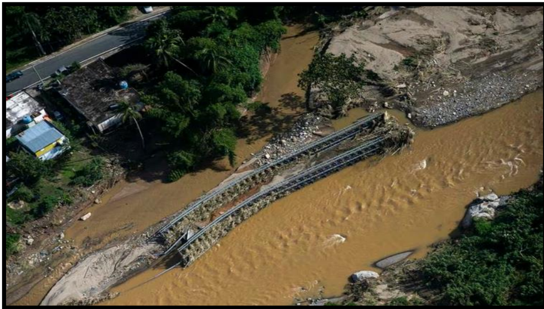
Figure 31: Infrastructure damage in the Municipality of Utuado. El Nuevo Día, September 22, 2022.
